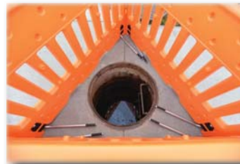
Protect Pedestrians From Work Zone Hazards
