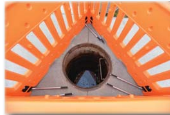
Protect Pedestrians From Work Zone Hazards
